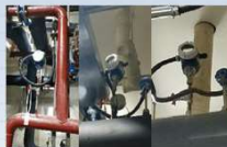
Circulating Water Metering
