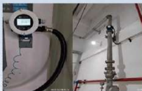
Landfill Leachate Metering
