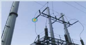
Partial Discharging Monitoring
