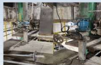
Washing Machine Inlet Metering
